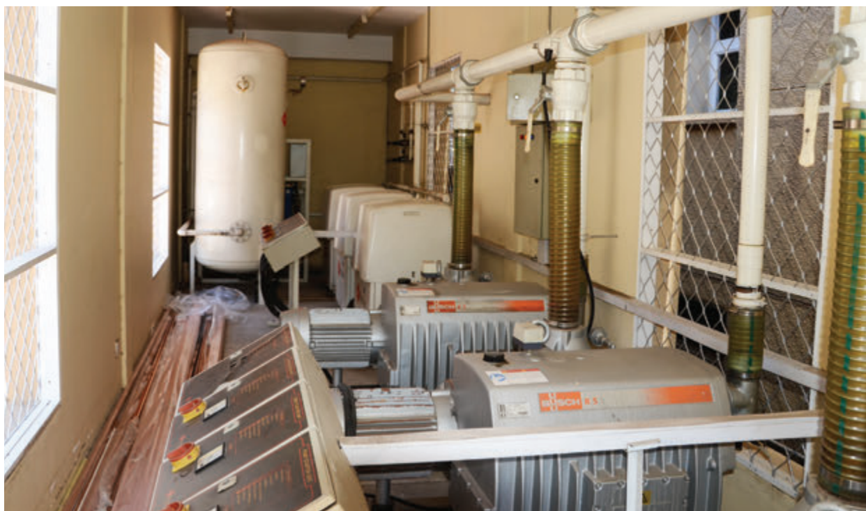
Alterations Done to Compressor Room to Increase Energy Efficiency
